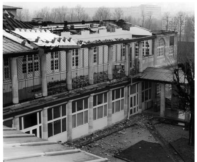
Fig. 2 Esquirol Hospital, building E with storm damage
