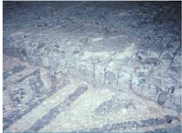
Fig. 12. Removal of cement mortar from the back of a pavement, by mechanical incisions, and working with a hammer and chisel
