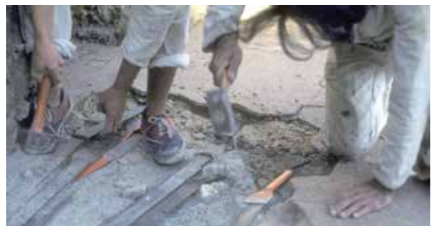
Fig. 11. Undercutting a pavement with iron bars, requiring great skill and judgement to prevent damage
