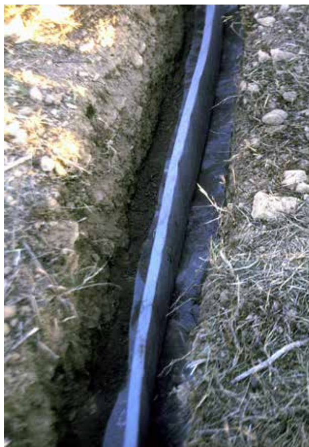
Fig. 8. Example of a geodrain installed on an archaeological site
