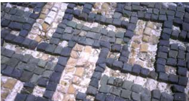
Fig. 4. Preferential erosion of white limestone tesserae by soluble salts from the ground
