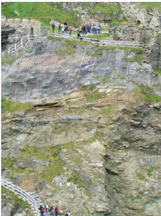
Fig. 5. Metal containment nets are one method employed to retain unstable rock slopes, as on this mediaeval site of Tintagel, England (©Arthur McCallum – English Heritage)
